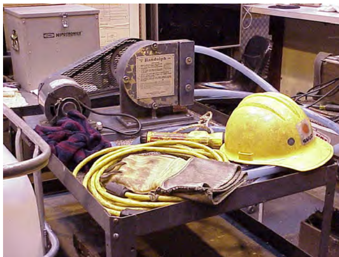
Figure 4: Example of a portable pumping system used by SMUD to move the FR3™ fluid around the transformer shop.
