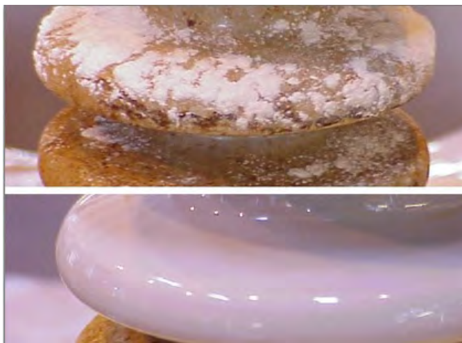
Figure 6: A bushing covered in polymerized ester fluid at top. The same bushing after cleaning with vinegar and cream of tartar.
