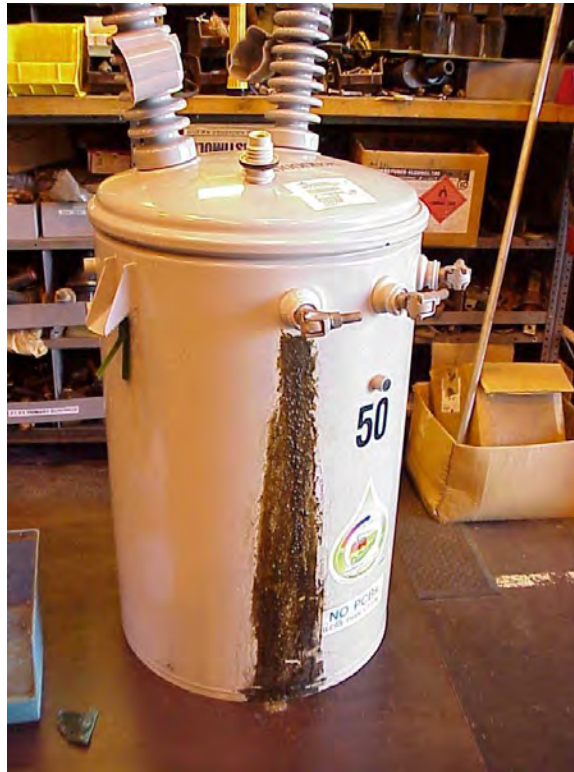
Figure 5: Polymerized ester fluid on the outside of a transformer tank.
