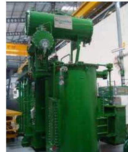
First power transformer with FR3 fluid for Tata Power
